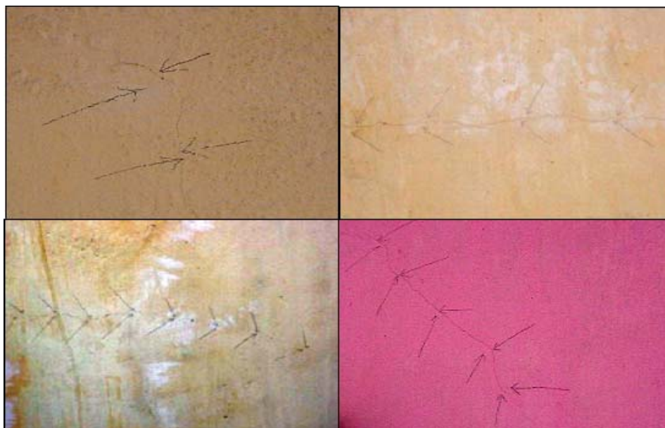
Photograph 9. Some views of the cosmetic cracks developed at the first floor of the RCC test structure on 29.03.2006 at Kusmunda Project.
