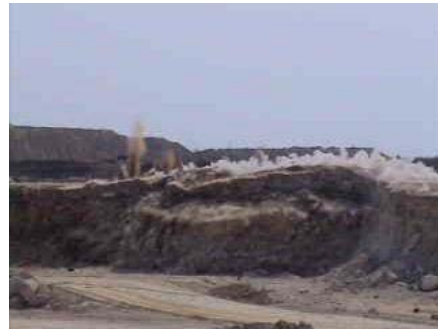
Photograph 3: Rock movement and excellent fragmentation due to bottom initiation at Ksumunda project.
