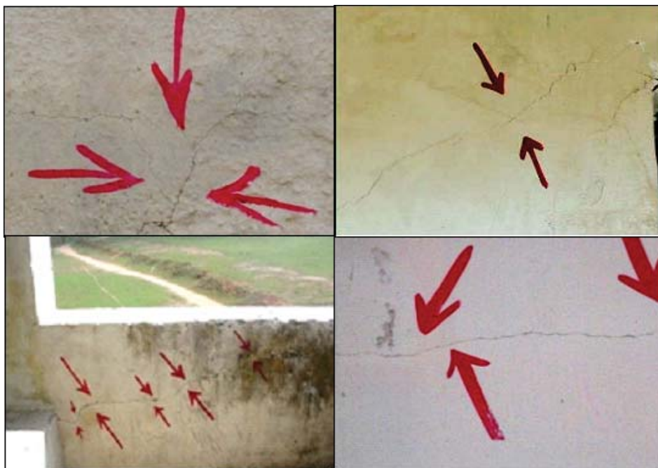
Photograph 6. View of the minor damage at the first floor of the RCC structure at Sonepur Bazari Project.
