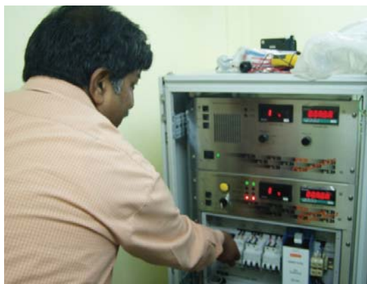
Figure 3: Phase I TTE Headend installation at Central Saunda
