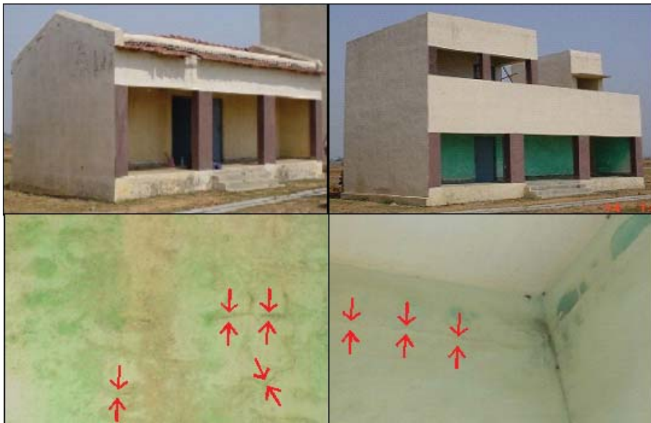
Photograph 5: The view of the cosmetic cracks developed in the brick-mud house and at the first floor of the RCC structures on 06.10.2004 at Sonepur Bazari Project.
