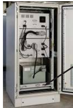
PLMT Unit shown in rear view of PED Headend Cabinet
