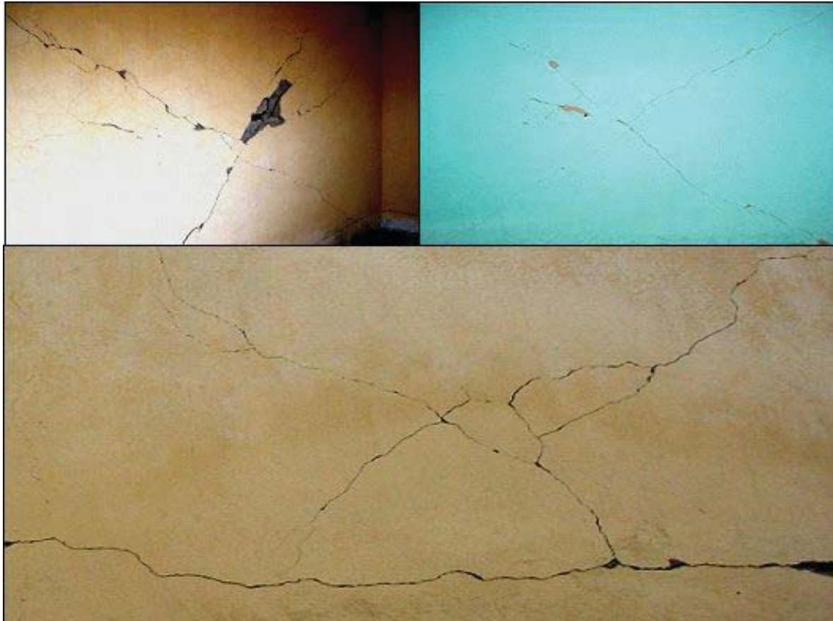
Photograph 11. Some views of the major damages developed in the first floor of the RCC structure on 10.05.2006 at Ksumunda Project.
