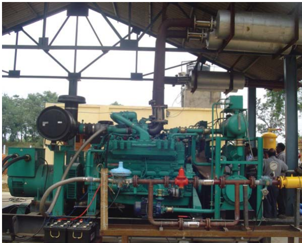
Fig 1: Gas based generators generating electricity at Moonidih
